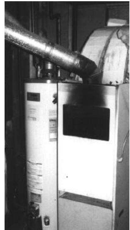
Flame roll-out is an indication of serious combustion problems. Some warning signs of flame roll-out include black or rusted areas in front of the burners (visible here), burnt wires and carbon deposits.
